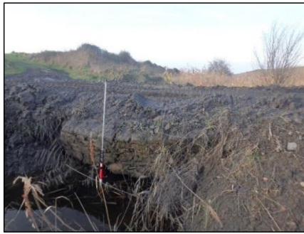
View 2: Upstream view of culvert crossing to the east of the Project road.
